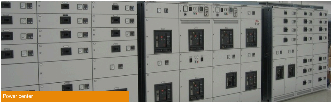
Turnkey electrical room in container
